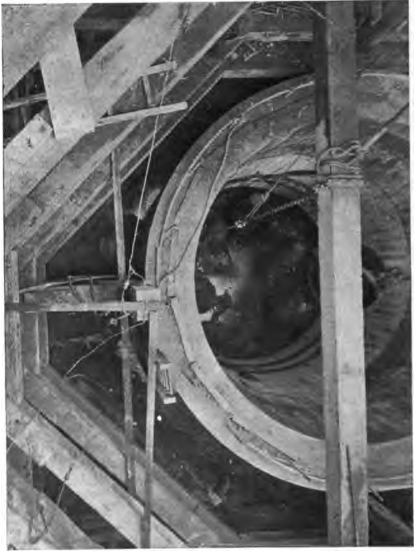
PLATE 209.—Contract 65. Shaft 7. Concrete Caisson Used to Reach Rock. This caisson was sunk in the open adjacent to Harlem R. R.
